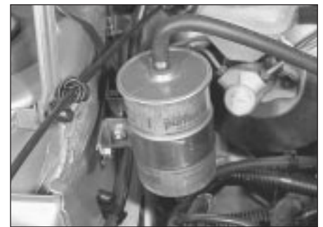
32.2 Fuel filter fuel hose and retaining clamp locations
