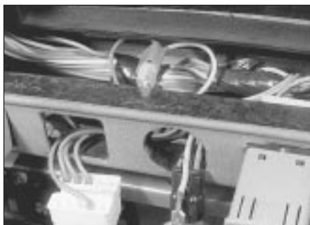
9.13 Heater control panel illumination light bulb (arrowed) on early models
